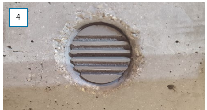
Stopper inside the concrete cone
